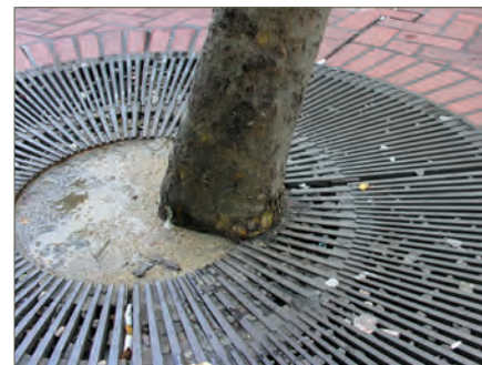
Settling off center - grate conflict
